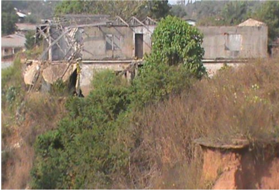
Fig. 10. A building damaged by gully in Auch
